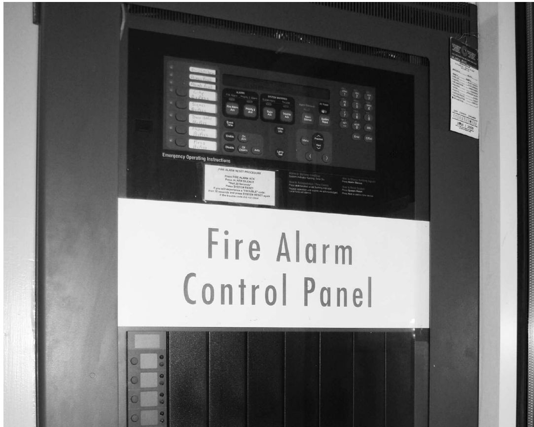
The fire alarm control panel inside of Santagati has gotten plenty of use this academic year
