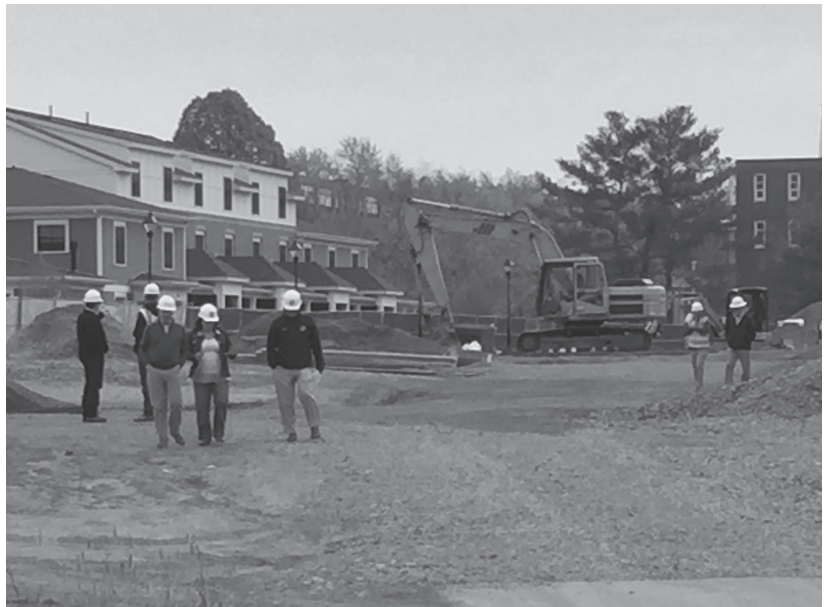
Work is progressing on the North Campus Pavilion, new home to the Girard School of Business.
